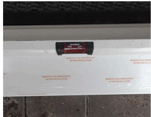
Ensuring the hinge side is slightly higher than the closing side, will give you a head start when toe and heeling the door.
