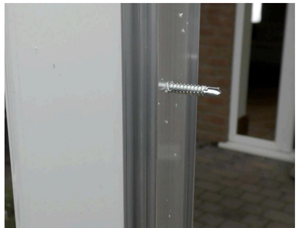
Place the door fixings to the door frame from the light glazing channel. This way no screw heads will be on show when the door is open.
