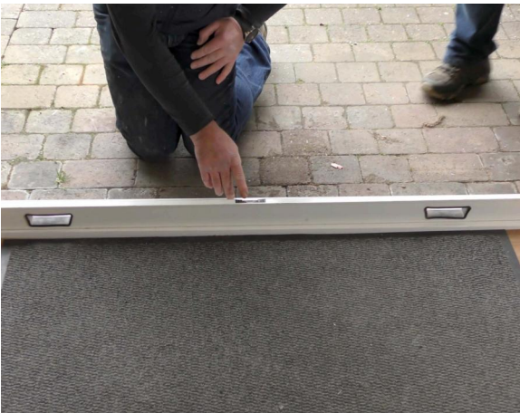
Place the cill on to the aperture. Use a spirit level to assess the level of the cill. If required, place packers under the cill, check the level and adjust if necessary.
