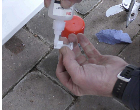
Attached the cill end caps using adhesive to seal and fix in place.
